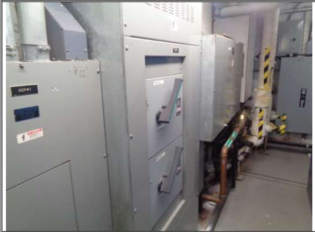
Photo 11 – View of electrical switch gear.
