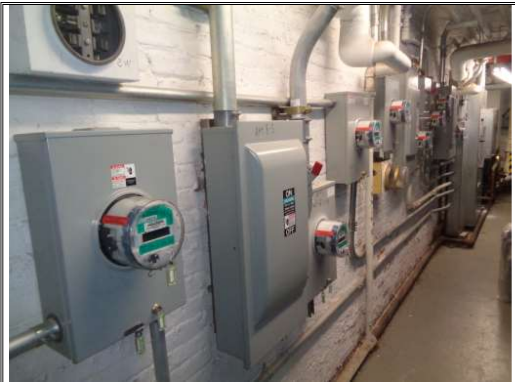
Photo 12 – View of electrical meters at the cellar.
