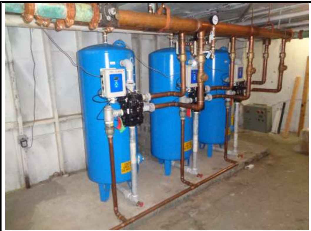
Photo 16 – View of the water pumps.
