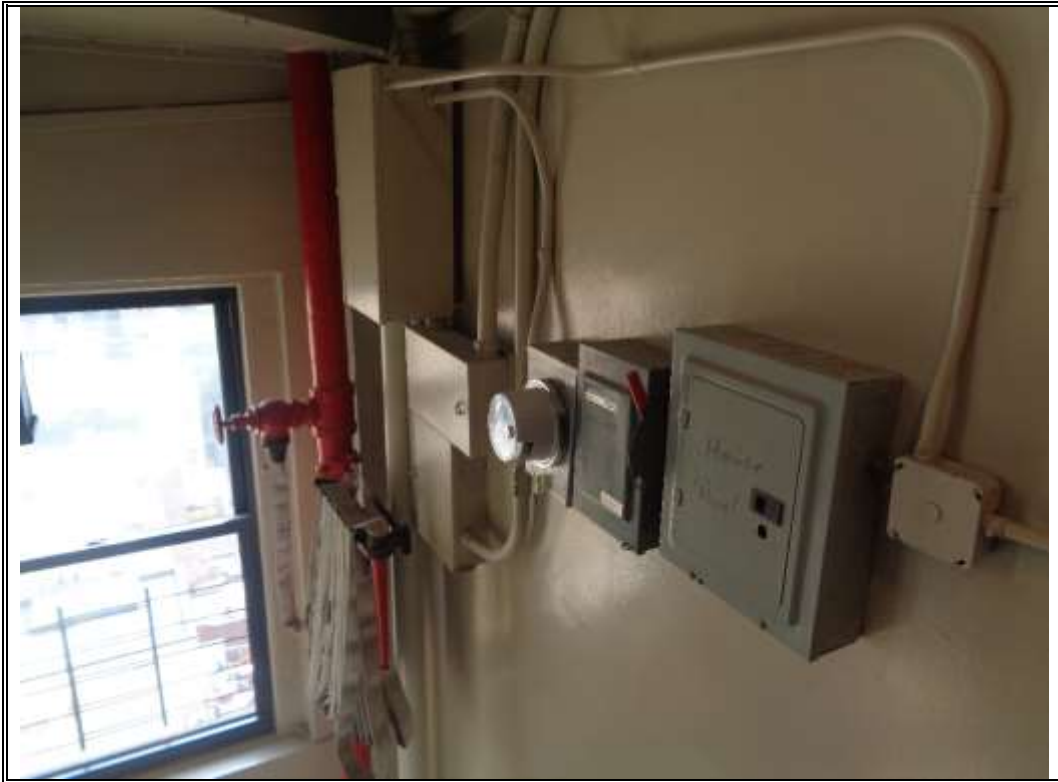
Photo 13 – View of electrical meter at the back stairs.
