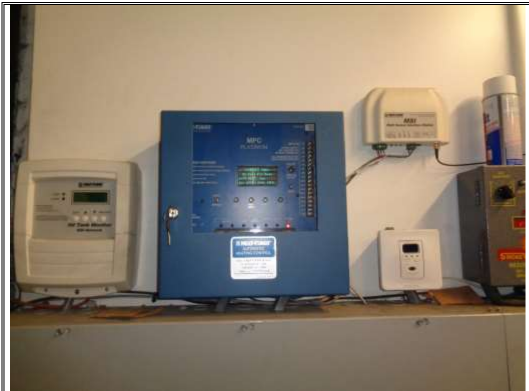
Photo 10 – View of the boiler controls.
