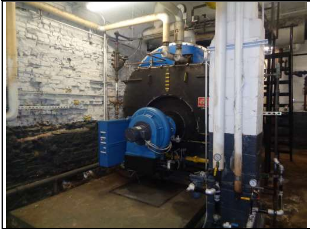
Photo 9 – Overall view of the boiler located in 40 East 83 rd Street.
