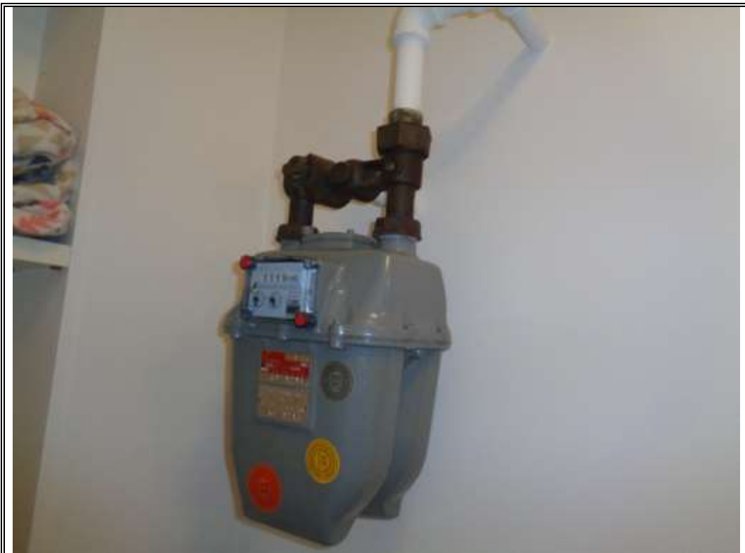
Photo 14 – View of a typical tenant gas meter.
