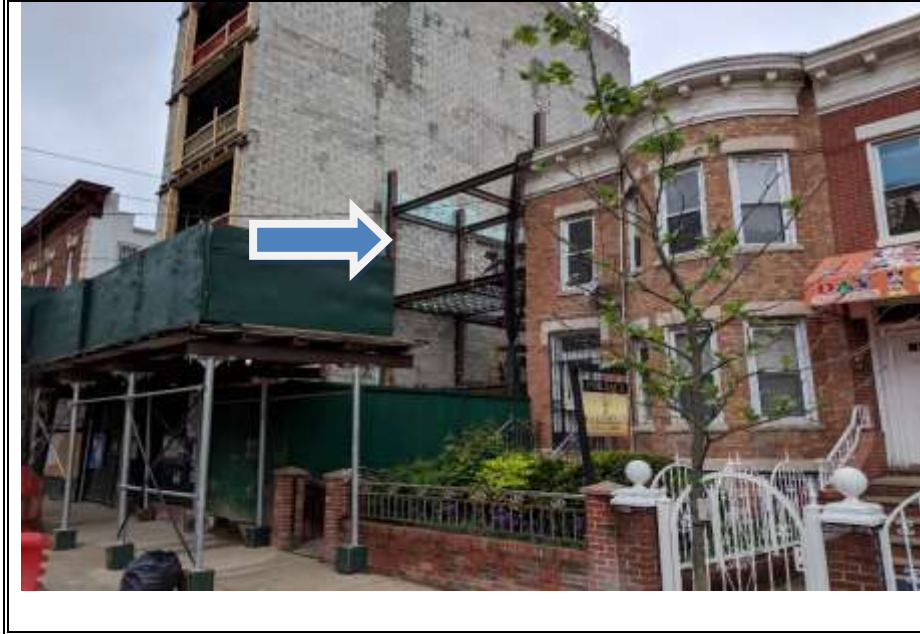
Photo 1 – View of the project. The subject project is the steel structure, not the masonry structure located at 371 Lincoln Road.
